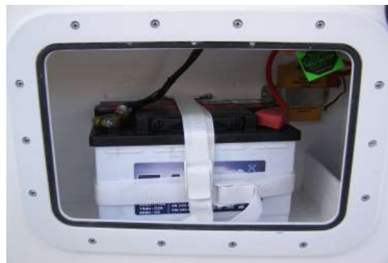
Opened hatch w/battery
